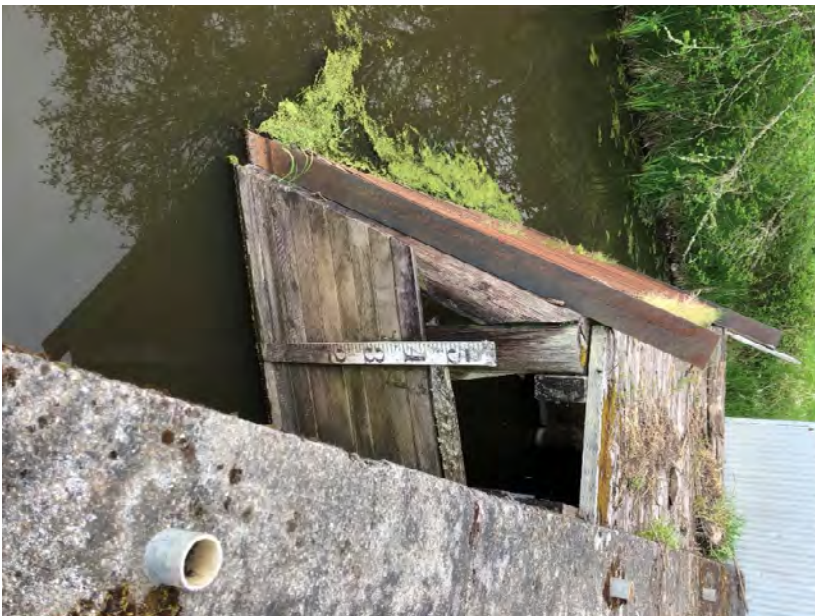
Staff Gage in pump station forebay
