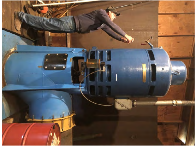
RDIC Pump Station – 200-hp Pump
