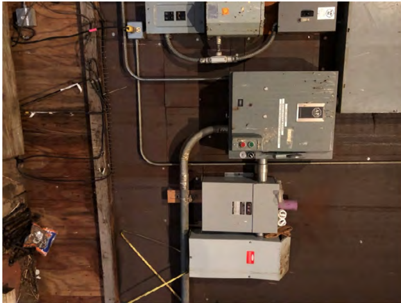
RDIC pump station – electrical panels
